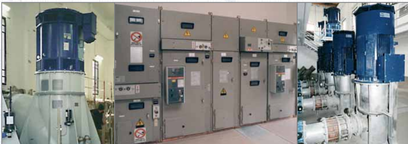
↑ one of the two 380 kW propeller electropumps
