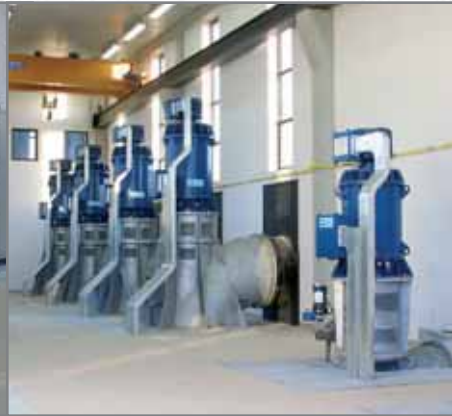
↑ pump room inside
