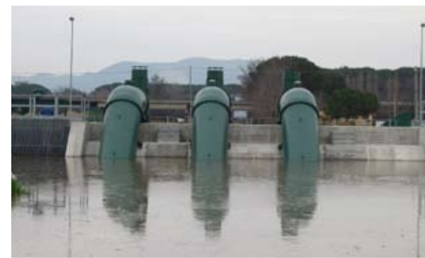
Consorzio di Bonifica Versilia Massaciuccoli Bufalina pumping station on the Napoleonic canal Amount of work € 689.774
