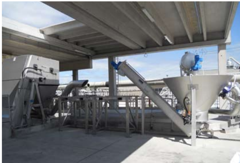
Acque del Chiampo S.p.A. Arzignano sewage treatment plant Amount of work € 548.961
