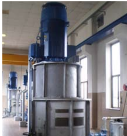
VERITAS S.p.A. Cà Emiliani pumping station Amount of work € 1.476.156
