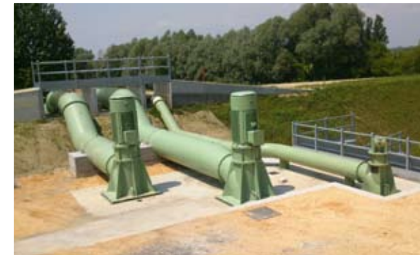
Municipality of Pordenone - Rugo di Valle, Rugo Noncello and Rugo dei Cucchi pumping stations Amount of work € 813.492
