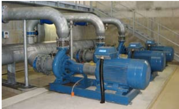
Associazione Irrigazione Est Sesia Dora pumping station Amount of work € 2.786.916
