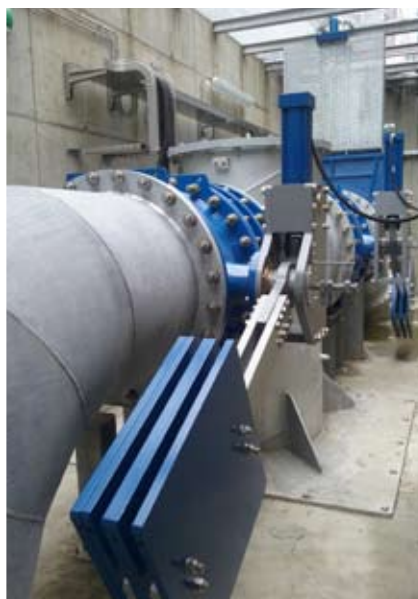
Consorzio della Bonifica Renana Expansion tank for Bagnetto plant Amount of work € 139.323
