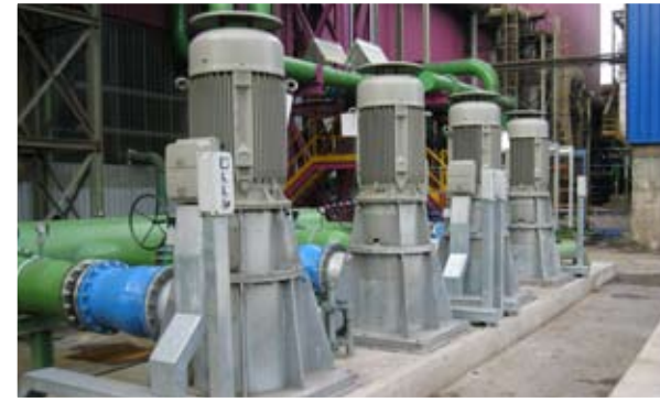
T.D. Supply of electric pumps for steelworks Amount of work € 760.365
