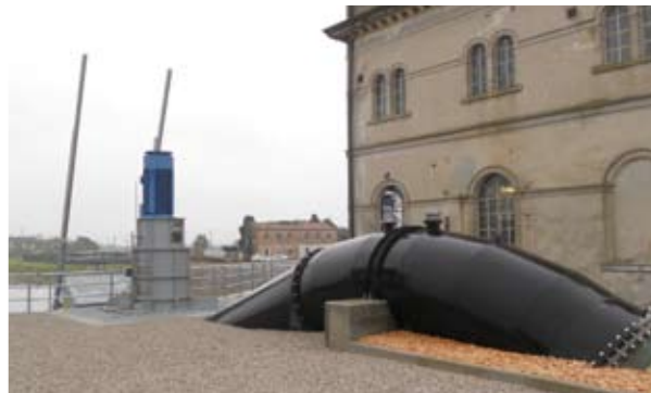
Consorzio di Bonifica Veneto Orientale Jesolo pumping station Amount of work € 439.199
