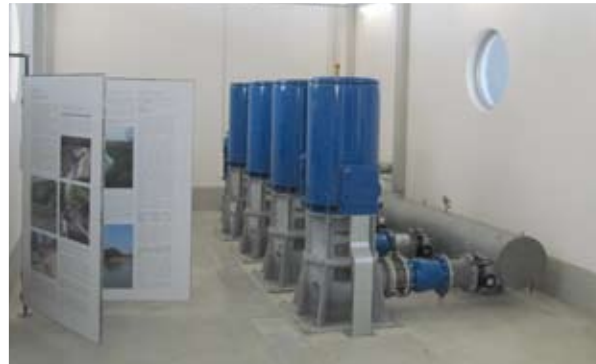
Consorzio della Bonifica Renana Medicina and Morella pumping station Amount of work € 768.000
