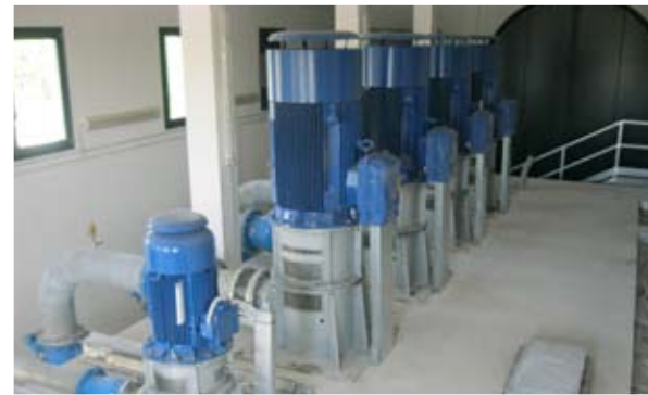
Consorzio di Bonifica Bassa Friulana Muzzana/Carlino pumping station Amount of work € 356.255
