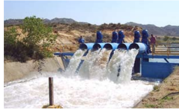
Bombas Ercole Marelli - Spain Supply of electric pumps (drought 2005) Amount of work € 602.000
