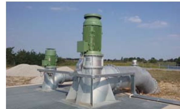
Consorzio di Bonifica Adige Euganeo Pascoletti pumping station Amount of work € 65.024
