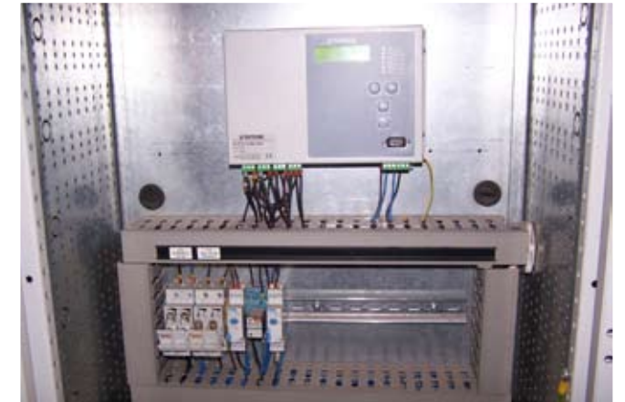
ETRA S.p.A. MV/LV technological adaptation at the Bassano waste plant Amount of work € 87.700
