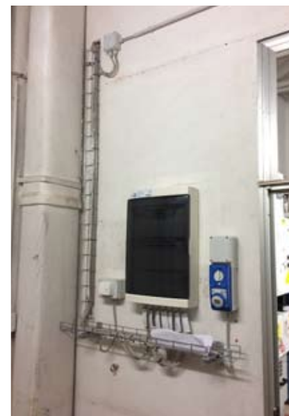
ETRA S.p.A. MV/LV cabin adjustment - Riviera Berica Amount of work € 79.635
