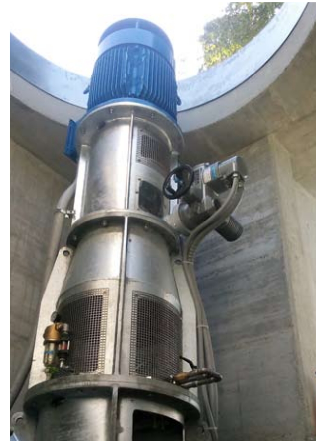
Consorzio di Bonifica della Romagna Occidentale Hydroelectric plant at Scodellino mill (biregulatory turbine) Amount of work € 116.289
