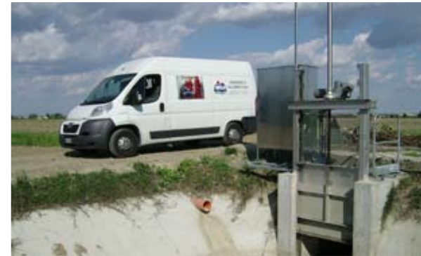
Consorzio della Bonifica Burana Automation of sluice gates of the consortium water network Amount of work € 263.335
