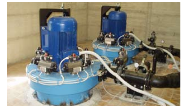
Municipality of Vinadio Neraissa hydroelectric station Amount of work € 158.565
