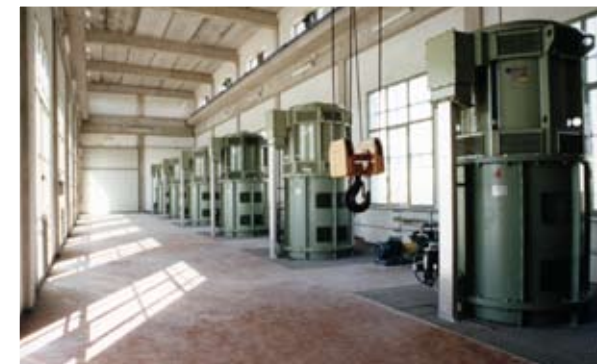
Consorzio di Bonifica Padana Polesana Bresparola pumping station Amount of work € 1.310.820
