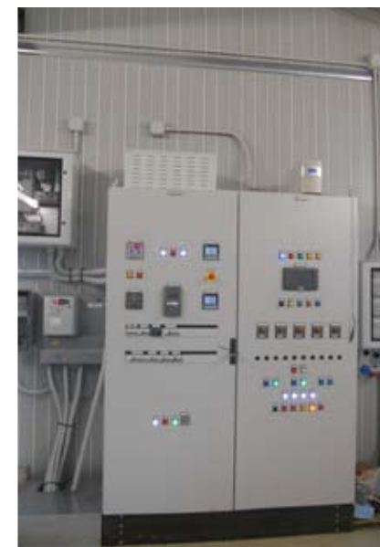
Consorzio di Bonifica Piave San Vito hydroelectric station Amount of work € 360.000
