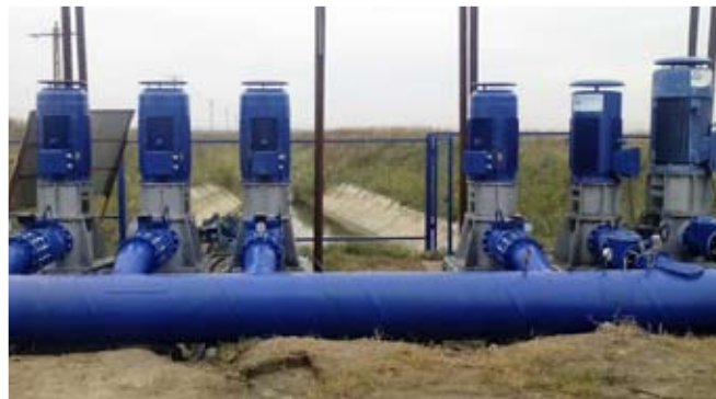
Private company - Romania Racovitã pumping station Amount of work € 164.250
