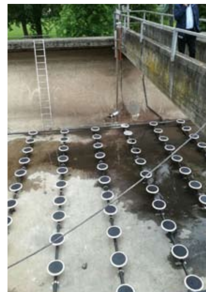
Livenza Tagliamento Acque S.p.A. Restructuring of Concordia Sagittaria sewage treatment plant Amount of work € 216.037
