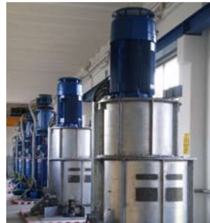
Consorzio di Bonifica Acque Risorgive Tessera pumping station Amount of work € 431.137
