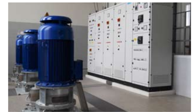
Consorzio di Bonifica Foce Isarco-Monte Vadena pumping station Amount of work € 344.748
