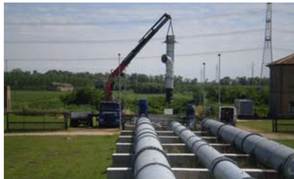
Consorzio di Bonifica Delta Po Adige Conca pumping station Amount of work € 443.715
