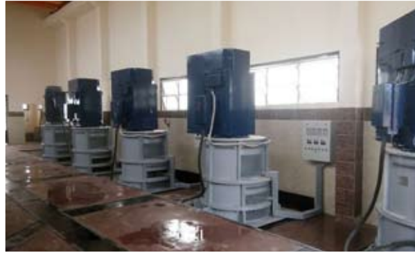
Ministry of Water Resources and Irrigation - Egypt Partial Rehabilitation of El-Thawra no. 2.4 Irrigation Pumping Stations Amount of work € 1.039.767
