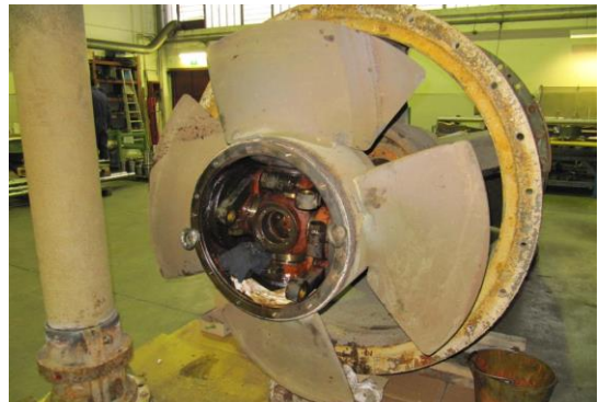
N. 1 electric-pump RIVA of 5500 l/sec H=5,5 rpm 368 Cartoccio pumping plant
